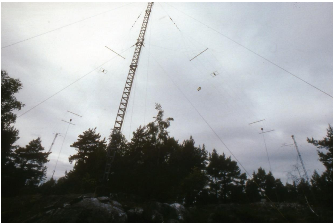
137. Kustradiostation mottagardel. Bredbandsdipoler
